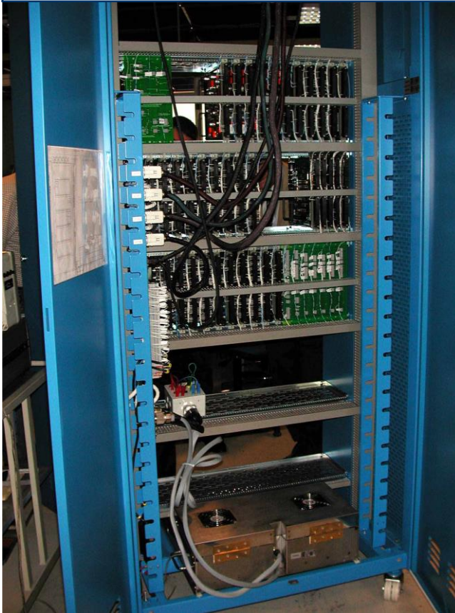
PA (Automatic Pilot) Cabinet
