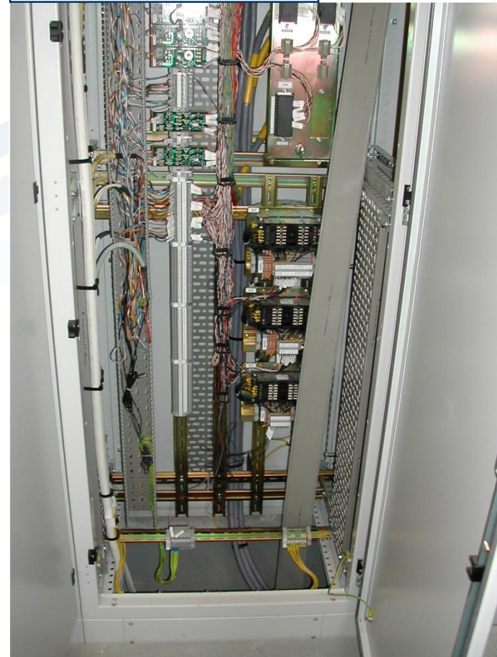
Cable Distribution Panel
